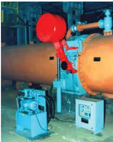
Penstock protection valve with bypass arrangement
